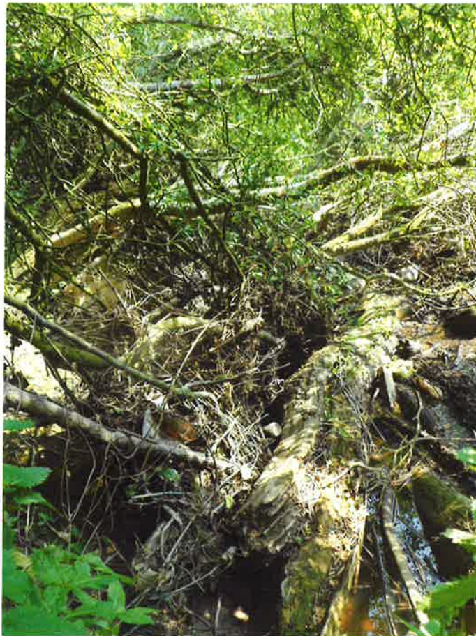
Burstow Stream Blockage, before the men started work
